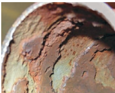
Corrosion in the form of rust and pipe-scale
