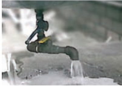
Untreated compressed air does not prevent large amounts of water from collecting in air receivers and downstream piping.
